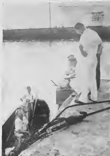
While the first pile is being driven for Finger Pier No. 2, T.S.D. engineers, right, check findings with N.H.W. men, left.
